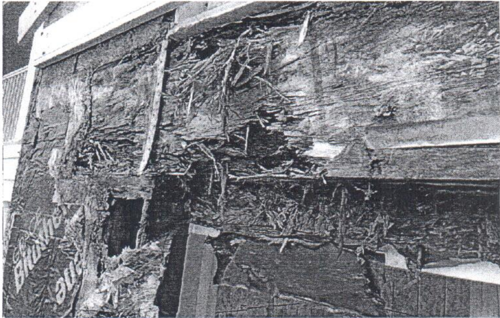
1FDE East Tower, 3rd Floor, East face. (See evidence sample)
