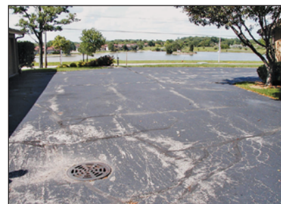
Light gray patches of asphalt show where sealcoat has been worn from the pavement. Applicators recommend reapplication of sealcoat from every 1 to 5 years. 1
