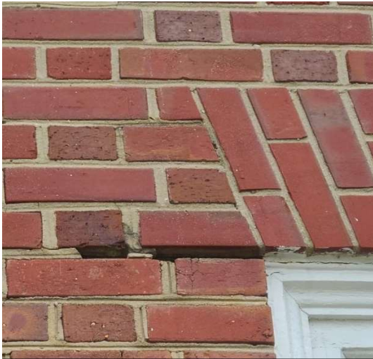
Wilson Hall – Deterioration of Brick allowing water intrusion.
