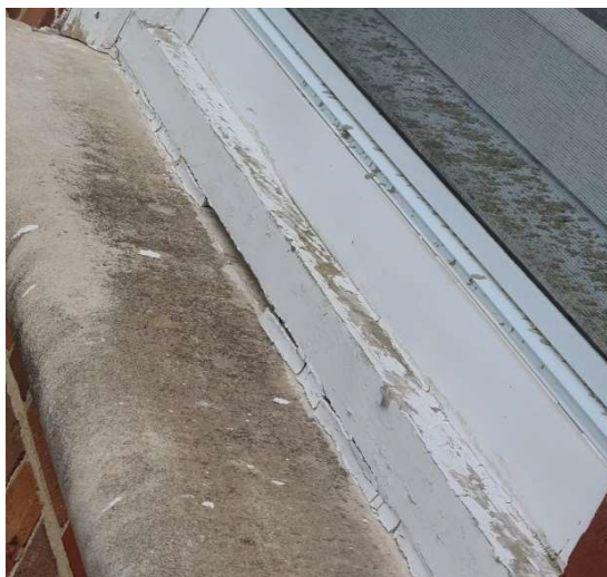
Wilson Hall – Deterioration of window allowing water intrusion
