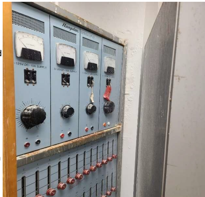
Water intrusion in electrical room
