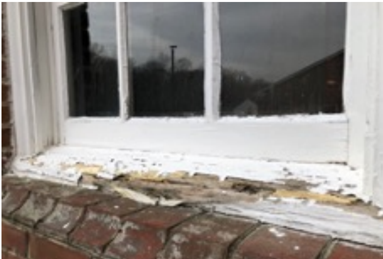
Carver Hall - Window deterioration and water intrusion
