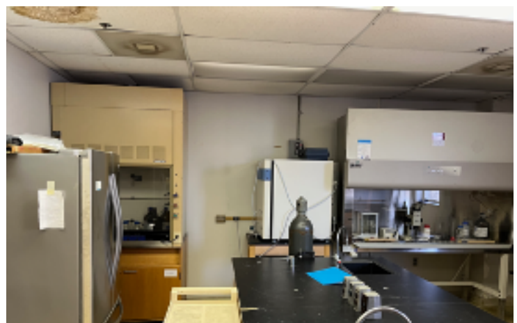
Research Lab in Carver Hall with water intrusion and mold
