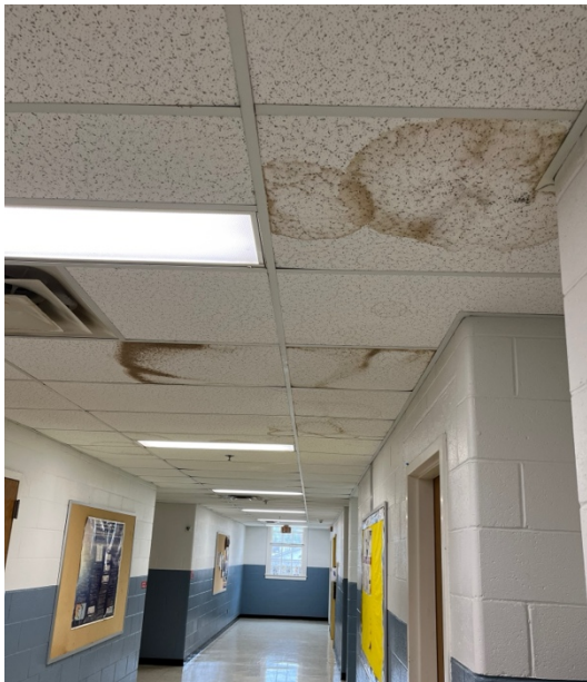
Carver Hall – water intrusion and issues of mold
