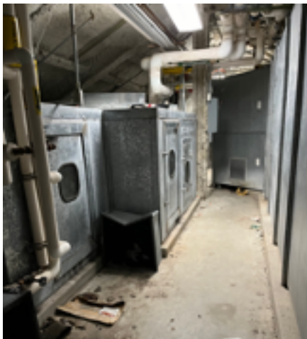
Antiquated HVAC unit in Carver Hall
