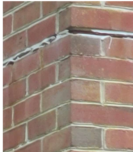
Exterior of Carver Hall; deterioration of brick
