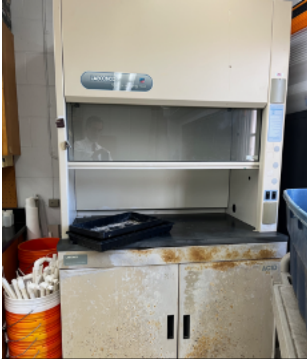
Antiquated Fume Hood with mold and damage from water intrusion
