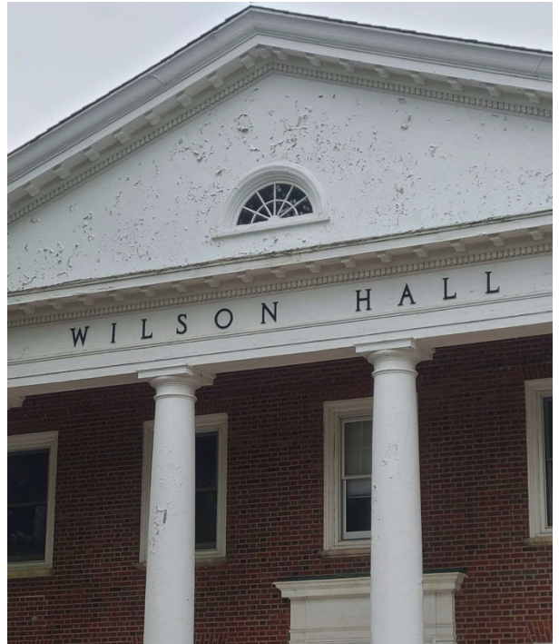
Wilson Hall - Deterioration of exterior facade
