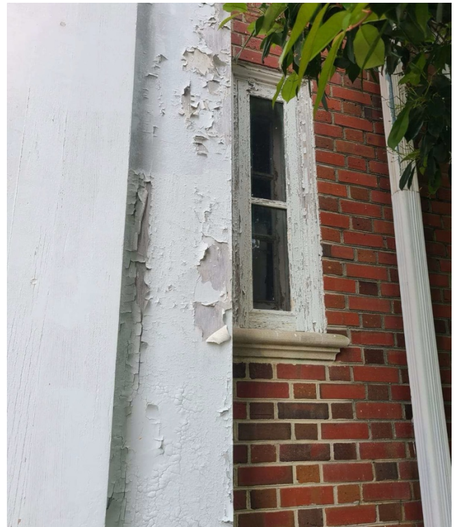
Trigg Hall – deterioration of window, brick and wood exterior
