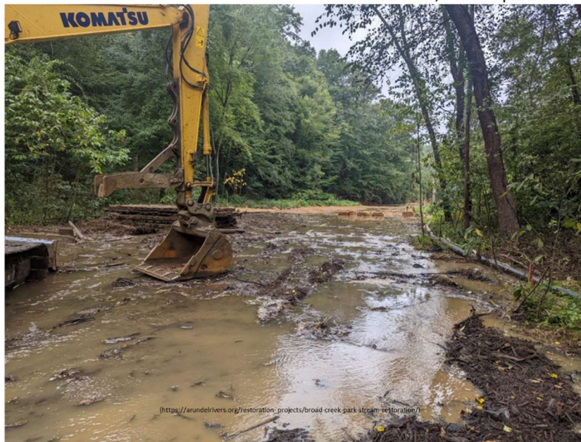
Broad Creek Park Stream "Restoration", Annapolis
