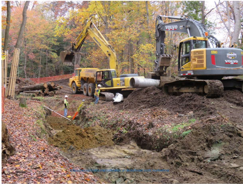
Broad Creek MVA Stream "Restoration," Annapolis
