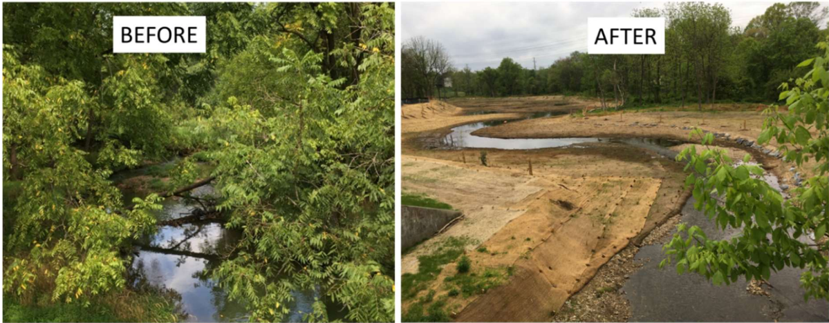
(Stream "restoration" in Blohm Park, Gaithersburg at Watkins Mill Rd. over Whetstone Run at the same location. Note the stream bank armor-plating on the right. (Left on 9/3/2020; right on 5/03/2021); by K.Bawer)
