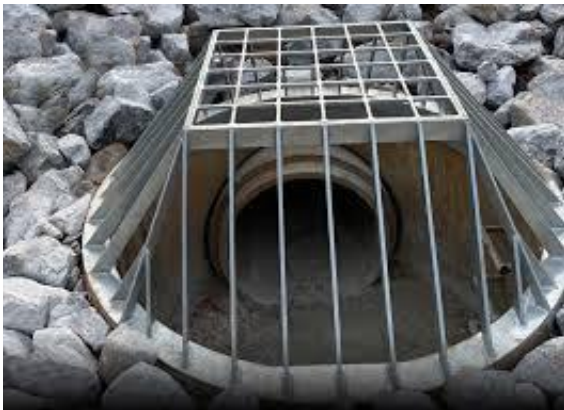
Trash Rack Inlet
