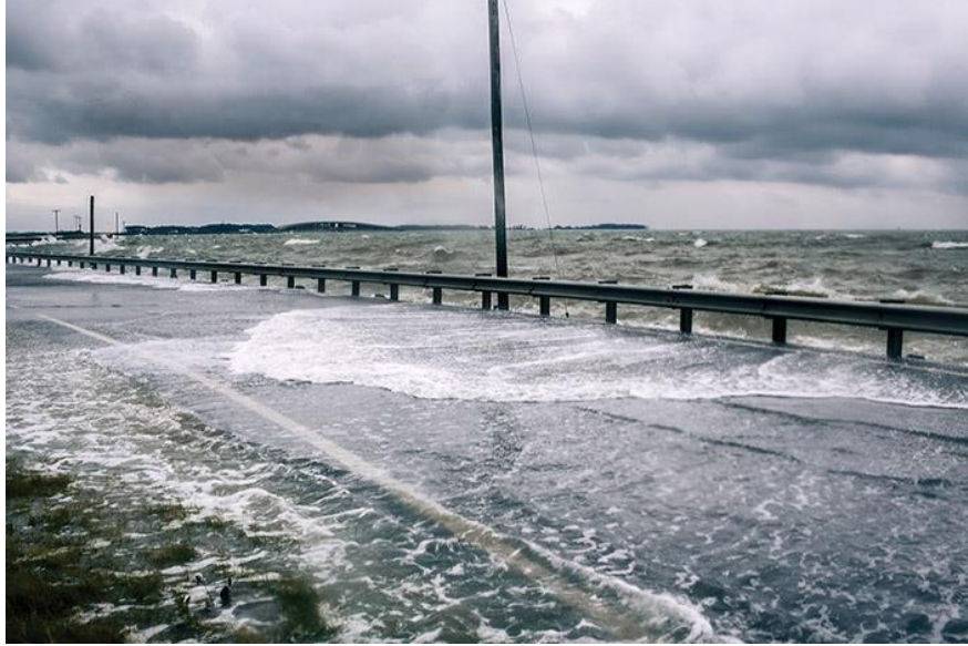
Flooded Hooper's Island Road Causeway; Photo from Baltimore Magazine
