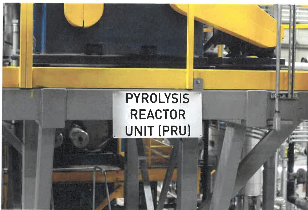
Pyrolysis equipment inside the Agilyx facility in Oregon. | Jared Paben/Resource Recycling, Inc.
