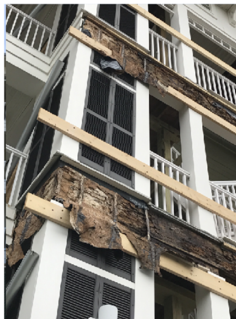
4FDE North Tower, degradation at return walls
