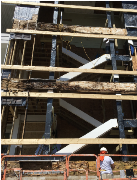
4FDE North Tower, Degradation of structural members at all levels
