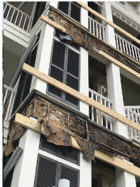
4FDE North Tower, degradation at return walls
