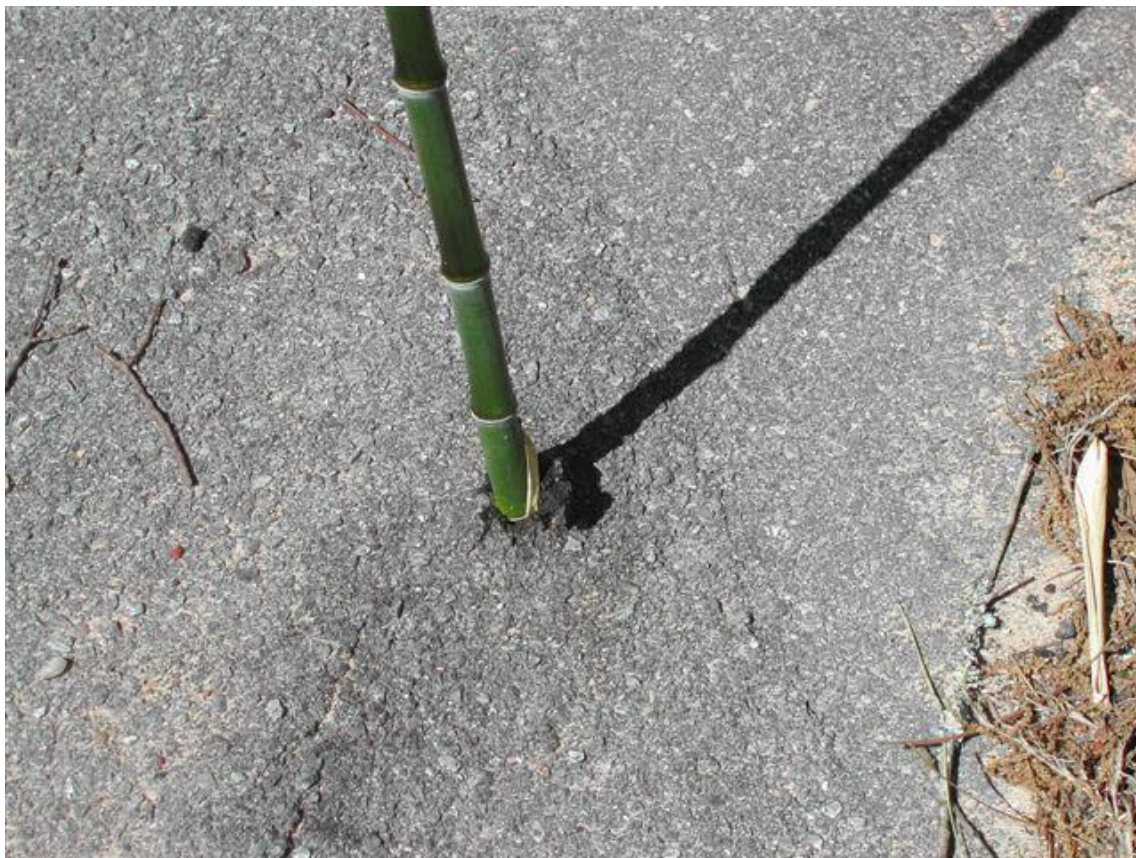
Invasive running bamboo stalk coming through asphalt from a rhizome (horizontal underground stem) that grew horizontally underneath the pavement from an adjacent bamboo grove
