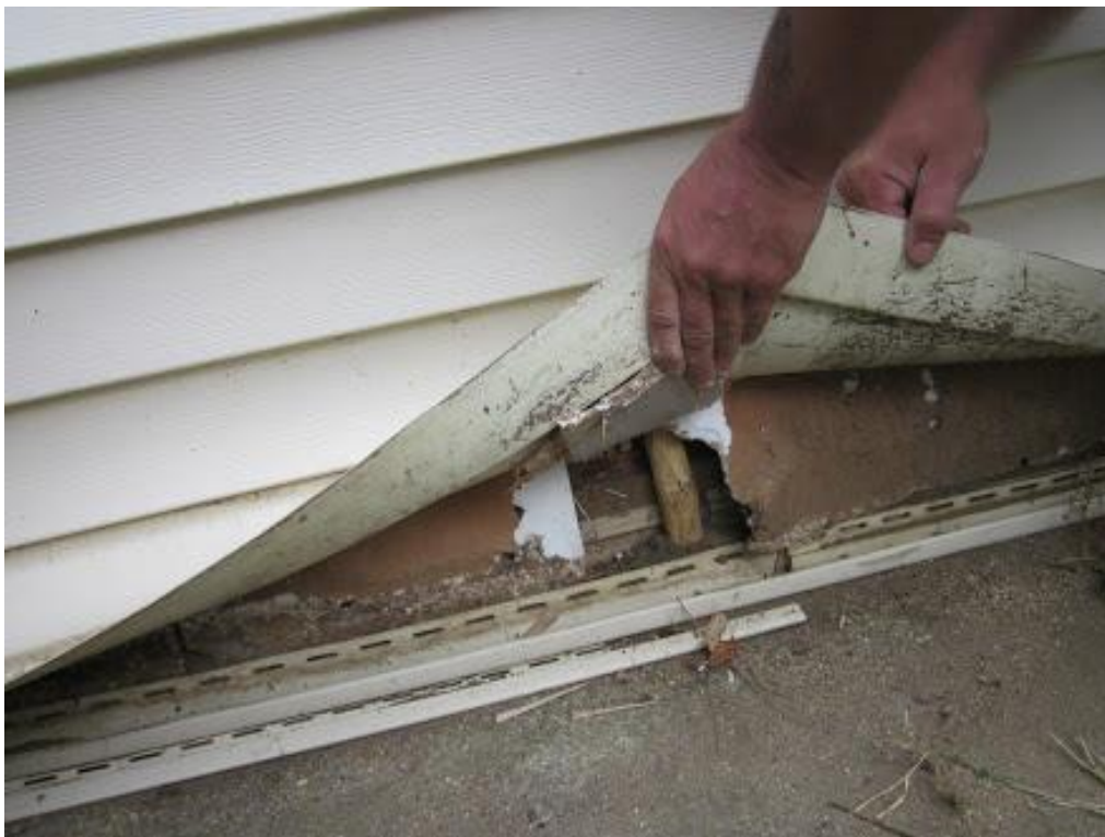
Invasive bamboo stalk growing behind sheathing and siding on a building
