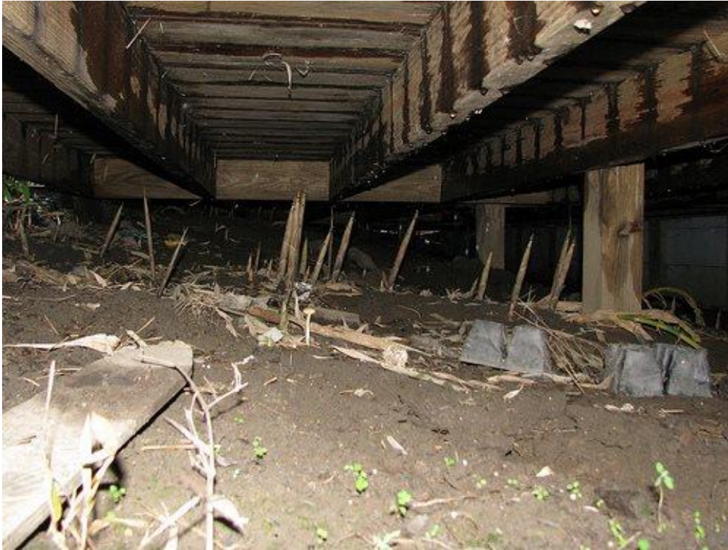
Stalks of invasive running bamboo sprouting into a crawlspace from underground rhizomes that spread horizontally in the soil from a bamboo grove
