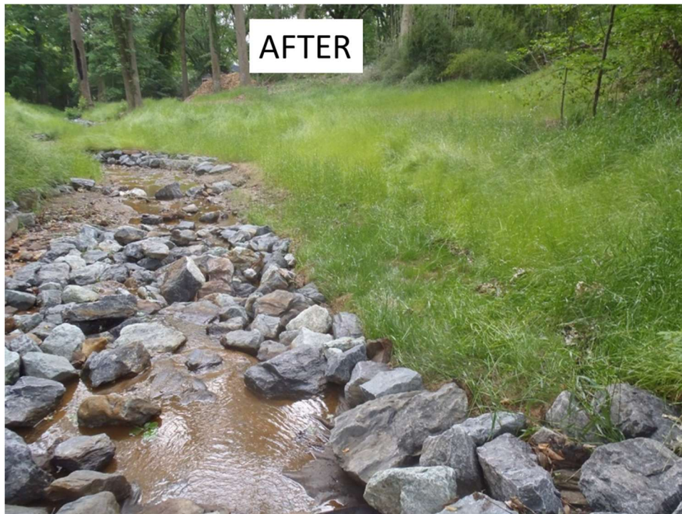
(Above: after construction, Takoma Branch, Takoma Park; photo by DPW, City of Takoma Park)
