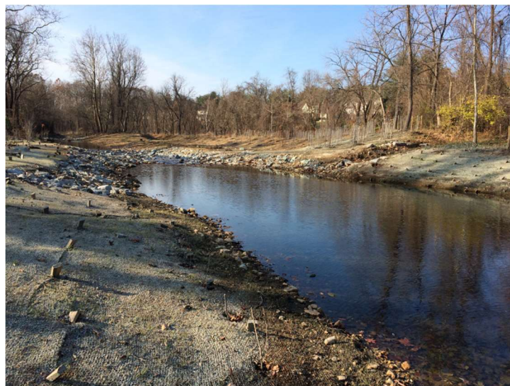
(Above: repair of the restoration in Lower Booze Creek, Potomac; photo by K. Bawer, 12/4/2021)
