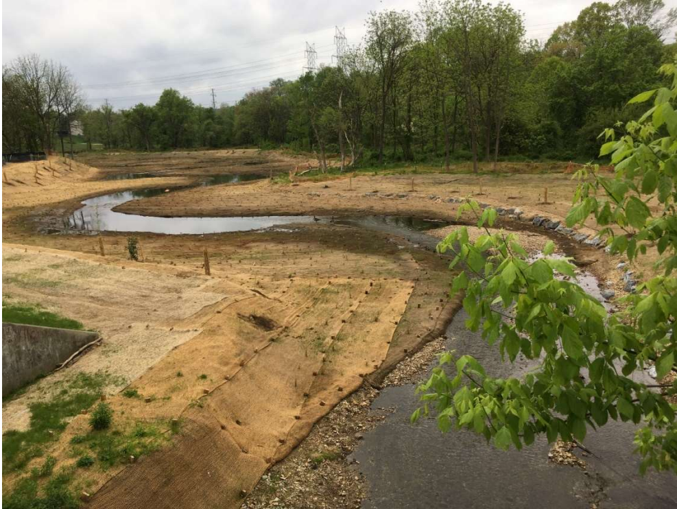
(Above: after construction: Whetstone Run in Blohm Park, Gaithersburg; by K. Bawer on 5/03/2021)
