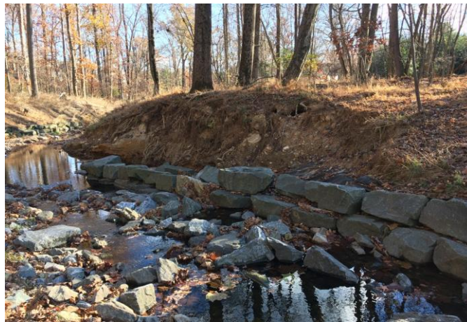
Exhibit 4: Stream restoration failure in Snakeden Branch, Potomac MD. Photo by K. Bawer
