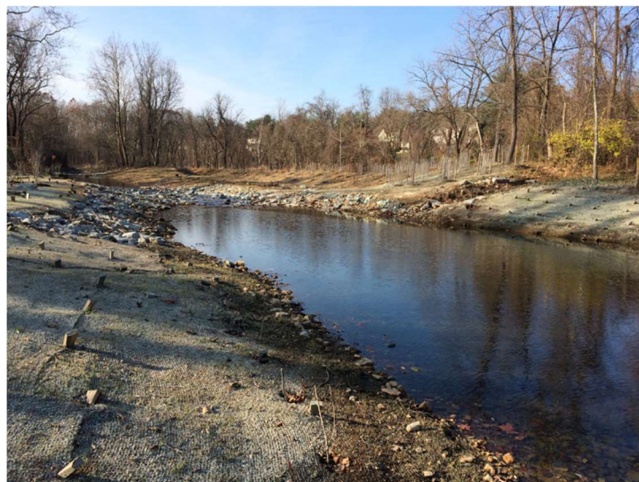
(Above: repair of the restoration in Lower Booze Creek, Potomac; photo by K. Bawer, 12/4/2021)
