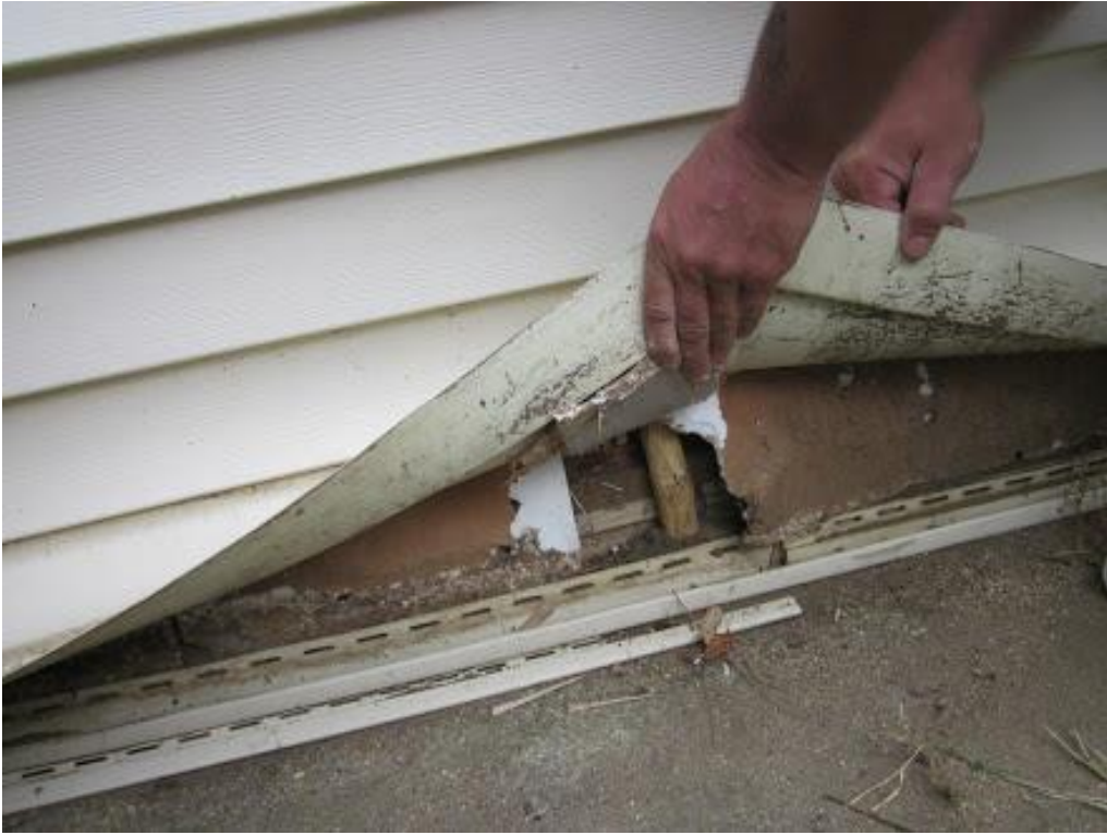
A stalk growing behind sheathing and siding on a building
