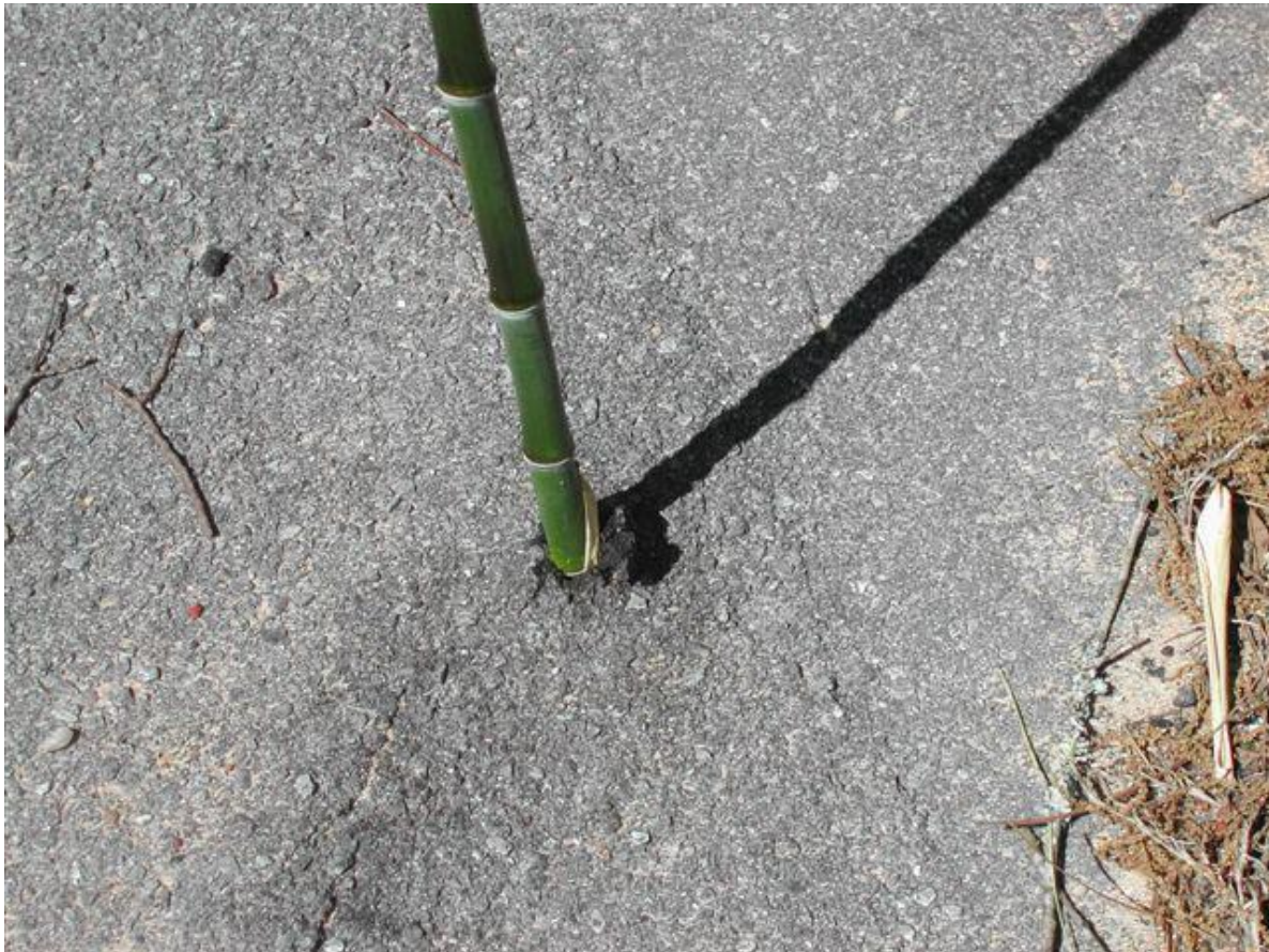
Invasive running bamboo stalk coming up through the asphalt because a rhizome (horizontal underground stem) grew horizontally underneath the pavement from an adjacent bamboo grove
