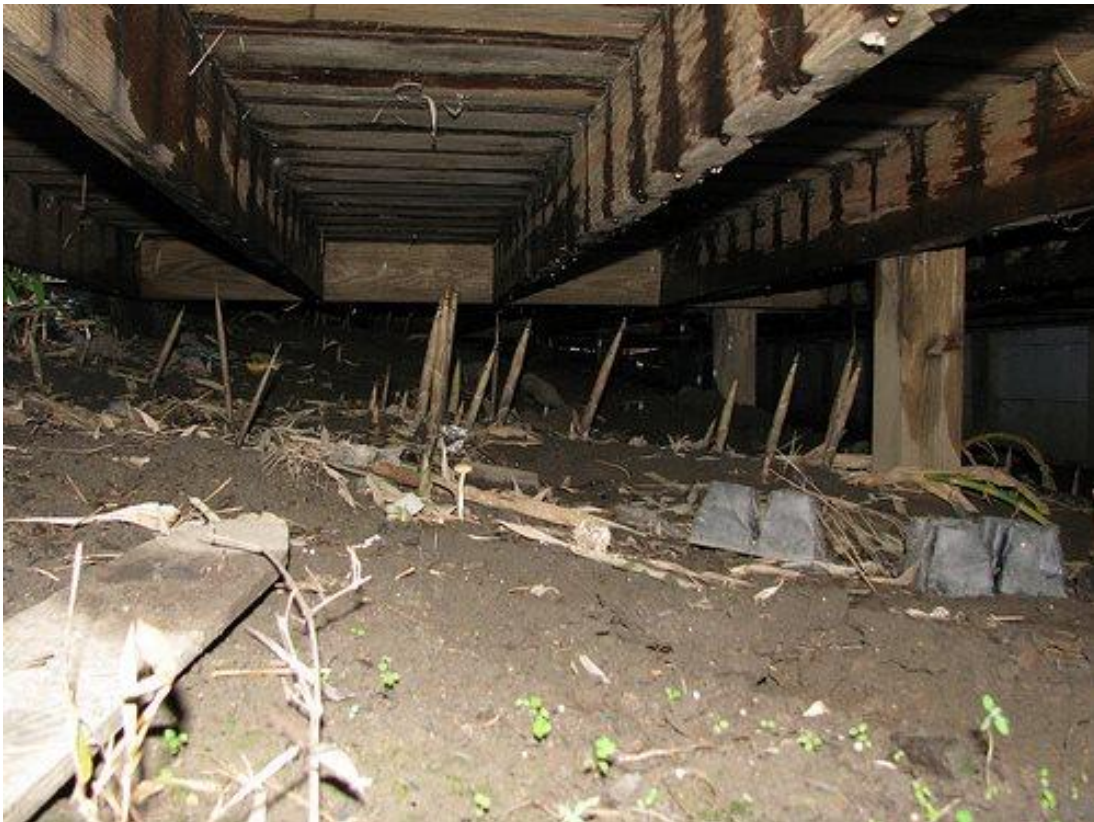
Stalks of running bamboo coming up from underground rhizomes that has grown horizontally under the soil beneath the building and are now visible in the crawlspace of a building
