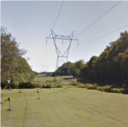
Existing 230 kV corridor
