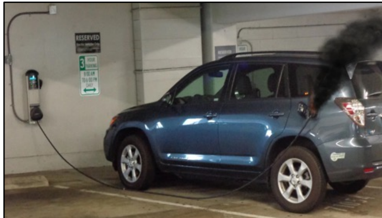
Figure 2. Note lack of power cut-off on <60A charger and lack of signage regarding where the circuit breaker is located.
