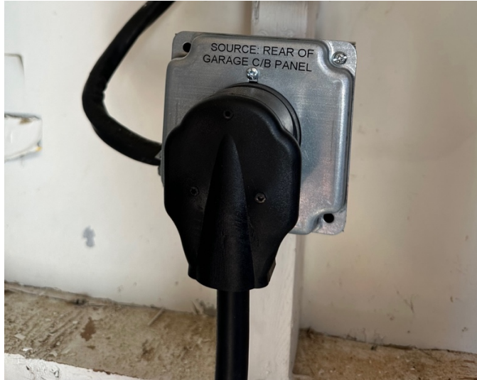
Figure 9. Home vehicle charging plug labeled for responders to know where to disable power.
