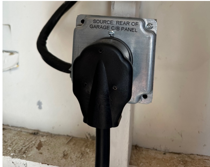
Figure 9. Home vehicle charging plug labeled for responders to know where to disable power.
