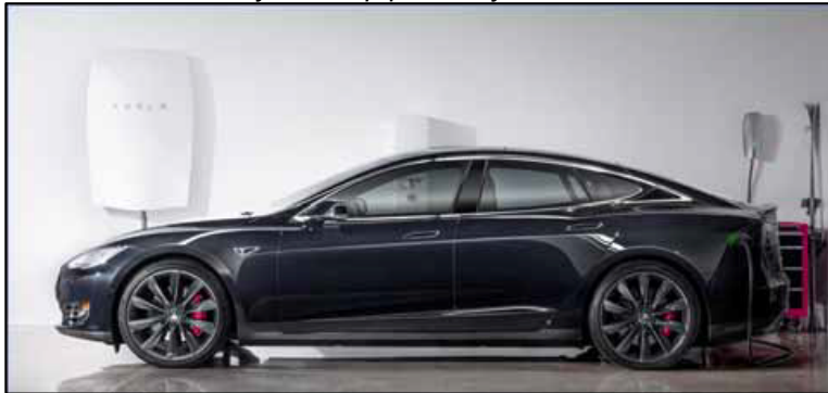
Figure 6. Garage Power Wall BESS visible above front of car.
