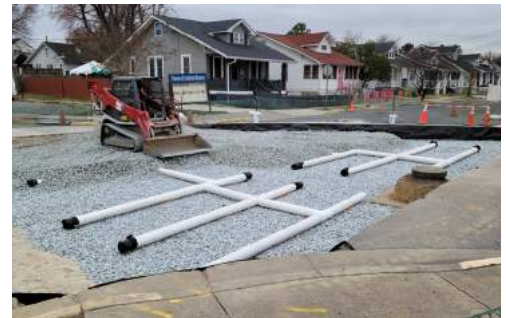
Placement of PaveDrain system including mid-drain (converted hydraulically to overdrain with standpipe)
