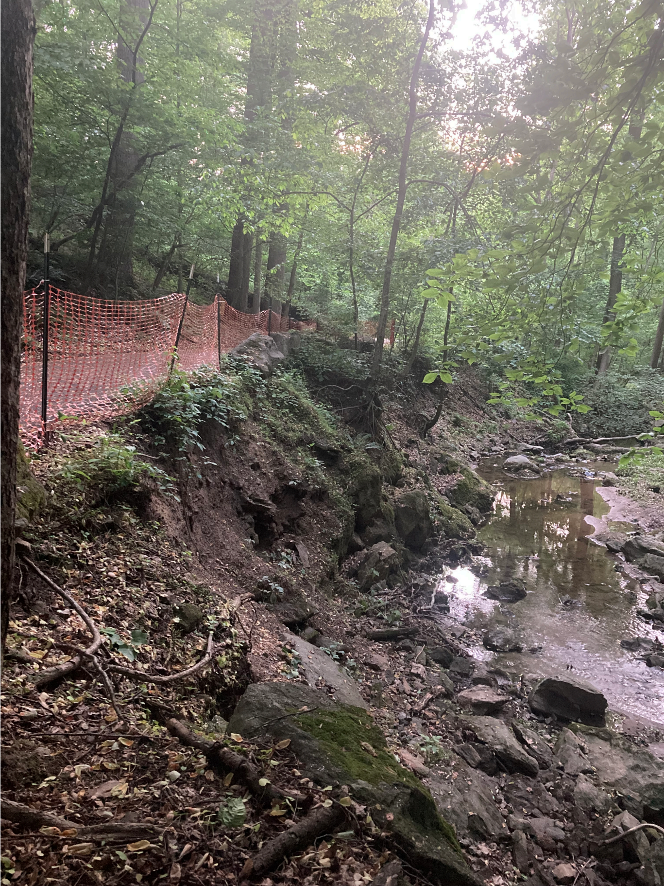
Exhibit 4 Cooper Branch erosion, Catonsville 2020
