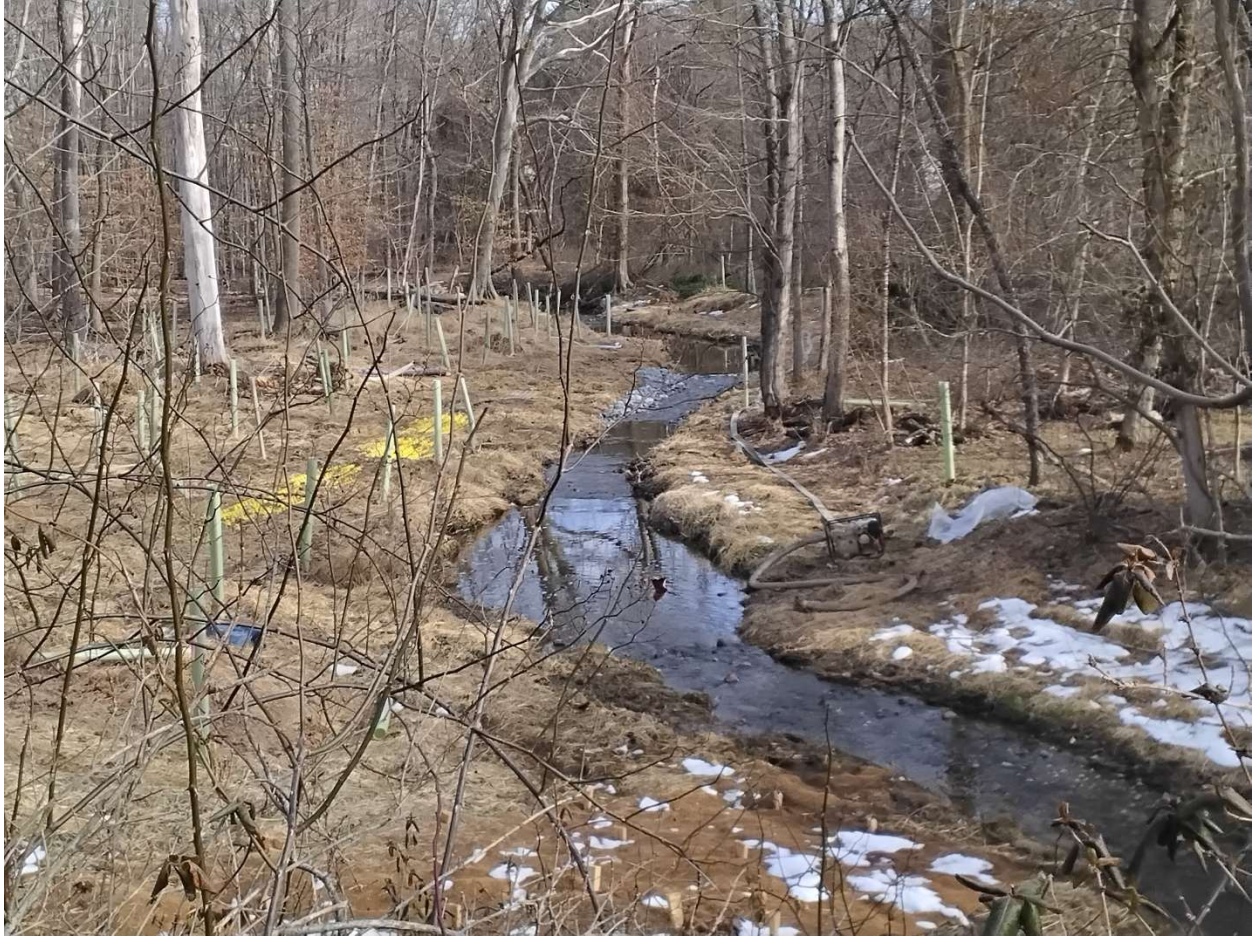
Here's the stream on 2/21/2026. The contractor will use the pump you see on the right - known as a "fish grinder" in the industry. They will pump the creek water out to be able to place more rocks along its banks. The stream never left its banks before the restoration. Photo s.boies
