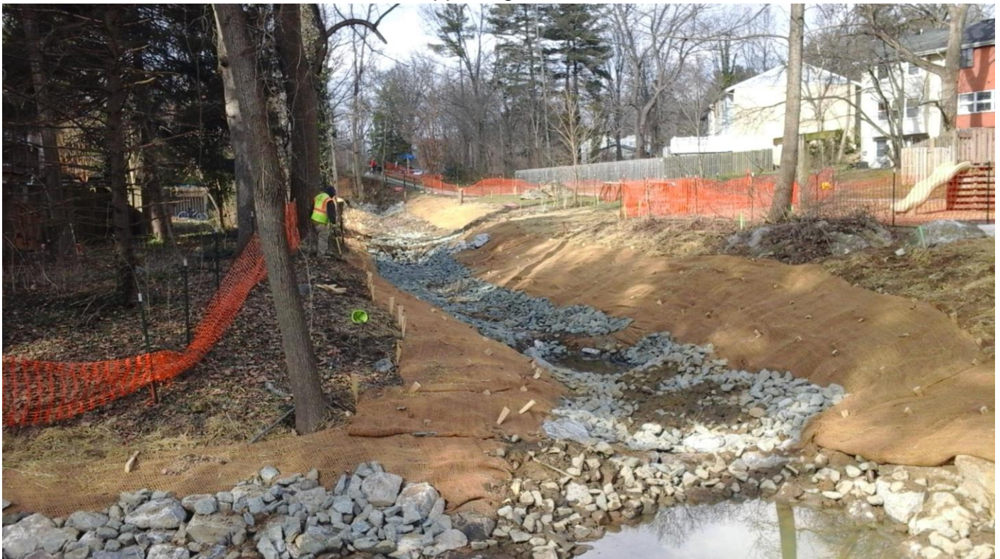
During Stream Restoration Work 4 – Natural benthic habitat is removed and replaced with new stream substrate material that is less effective for supporting diverse stream life.
