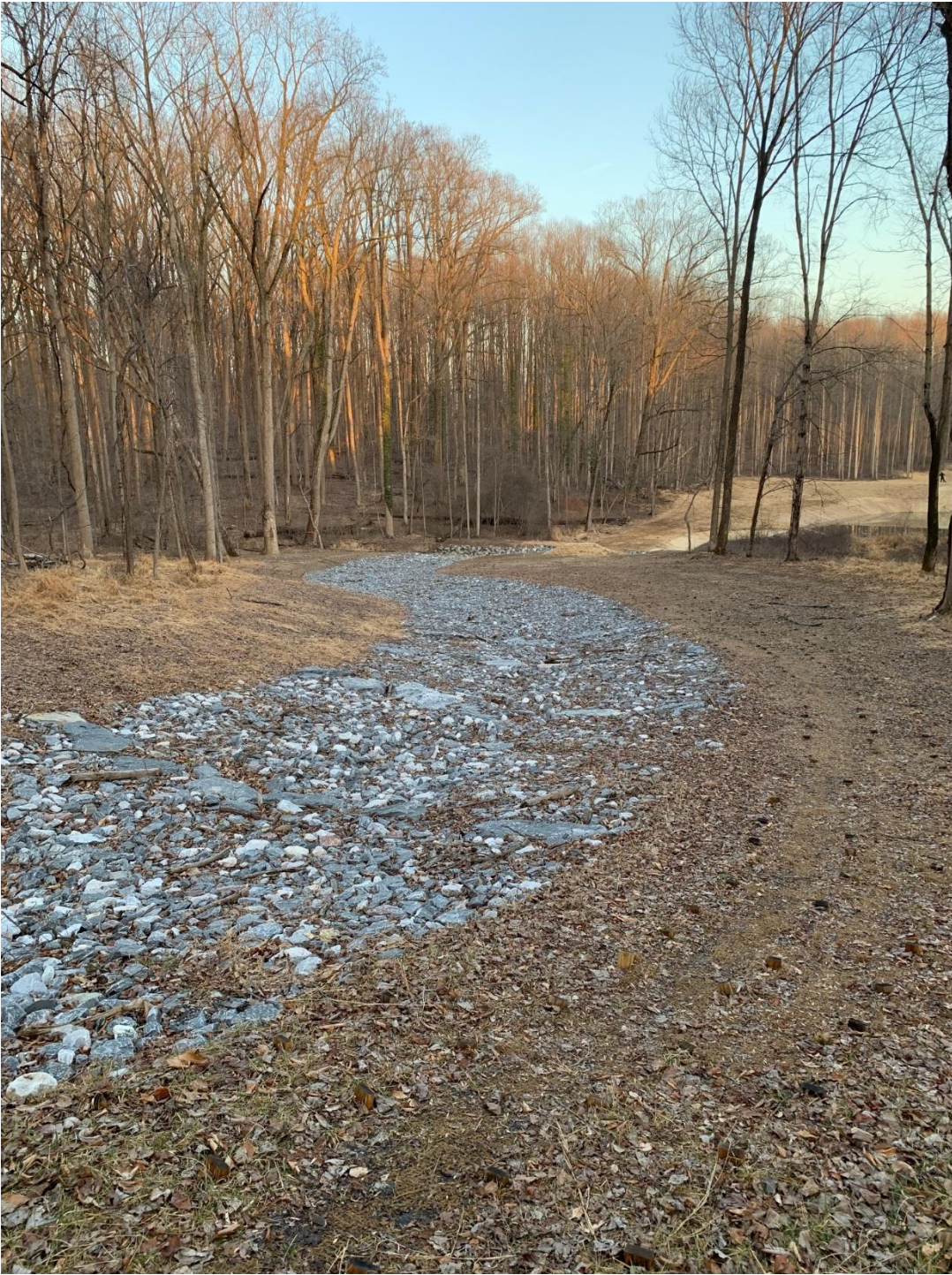
A whole woods was removed to install this gravel “stream restoration” which will heat the water before it reaches Centennial Lake.
