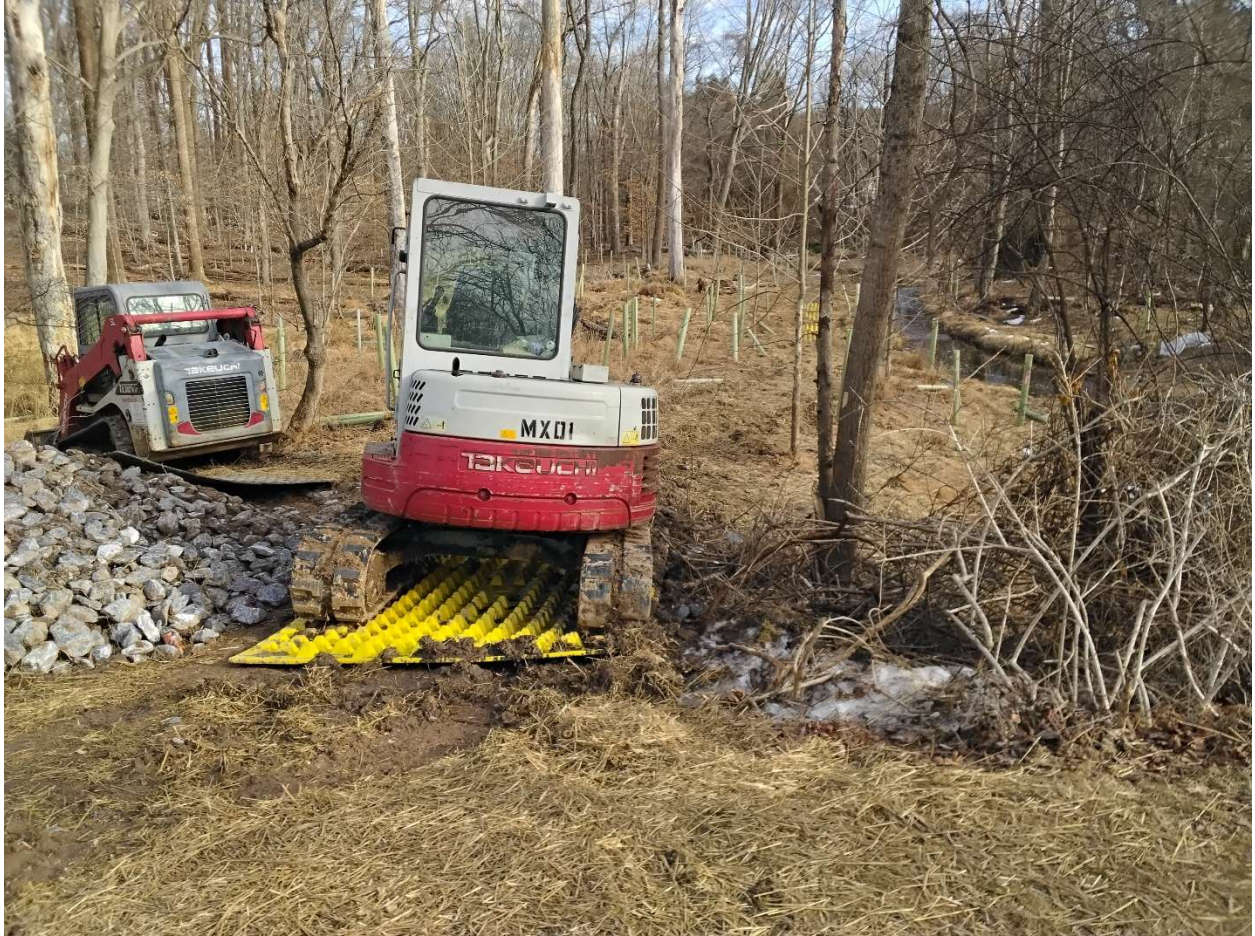
This is the same location on 2/21/2026 in year 6 of the restoration. This project cost our state 2.2 million dollars – just for credits for the SHA. Photo s.boies
