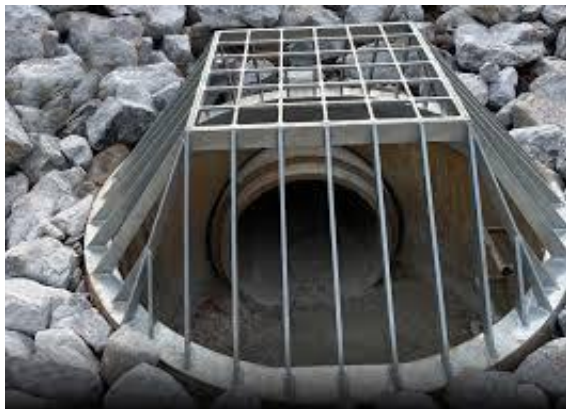
Trash Rack Inlet
