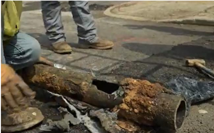
Cast iron pipe in Baltimore City
